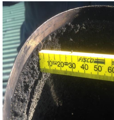
Coal dust 0.5mm thick on upper flue wall, 3 September
