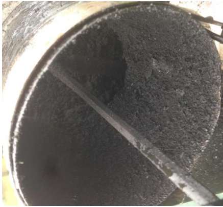
Black wood-coal soot, 4-10mm thick on upper flue wall, under 0.5mm on electrode, 27 June
