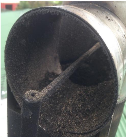
Black coal soot 1-4mm thick on upper flue wall, 0.1mm on electrode, 27 June
