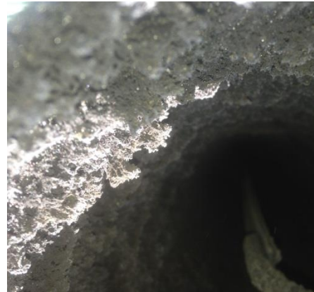
Light grey dust, 5-8mm thick on upper flue wall, 3 September
