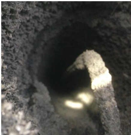
Wood-coal soot, less than \frac{1}{4} the distance between the lower flue wall and the bottom of the electrode, grey/black colour, 27 June
