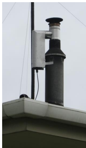
OekoTube circuit box on chimney
