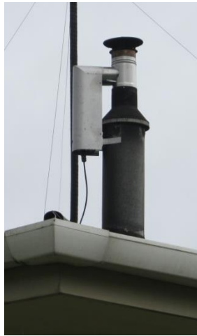
OekoTube circuit box on chimney
