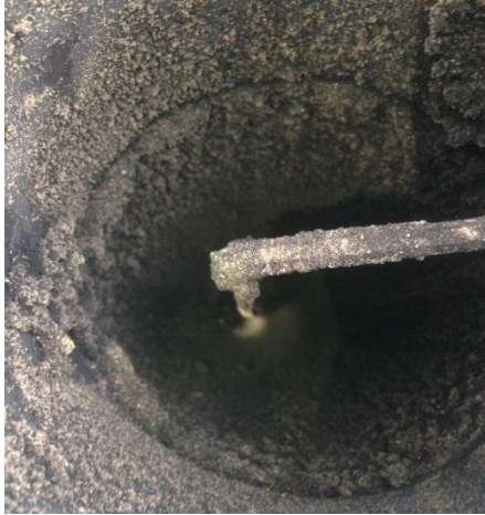
Lower flue wall, soot less than 19mm thick, 27 June
