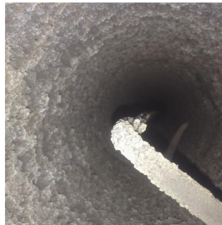
Light grey dust, approx. 5-8mm evenly spread on lower flue wall, 3 September
