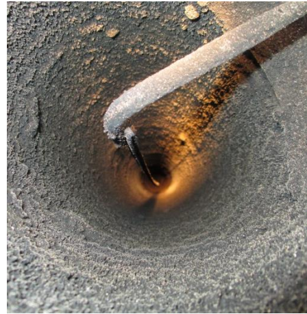
Lower flue wall, soot evenly spread, grey colour, 28 July
